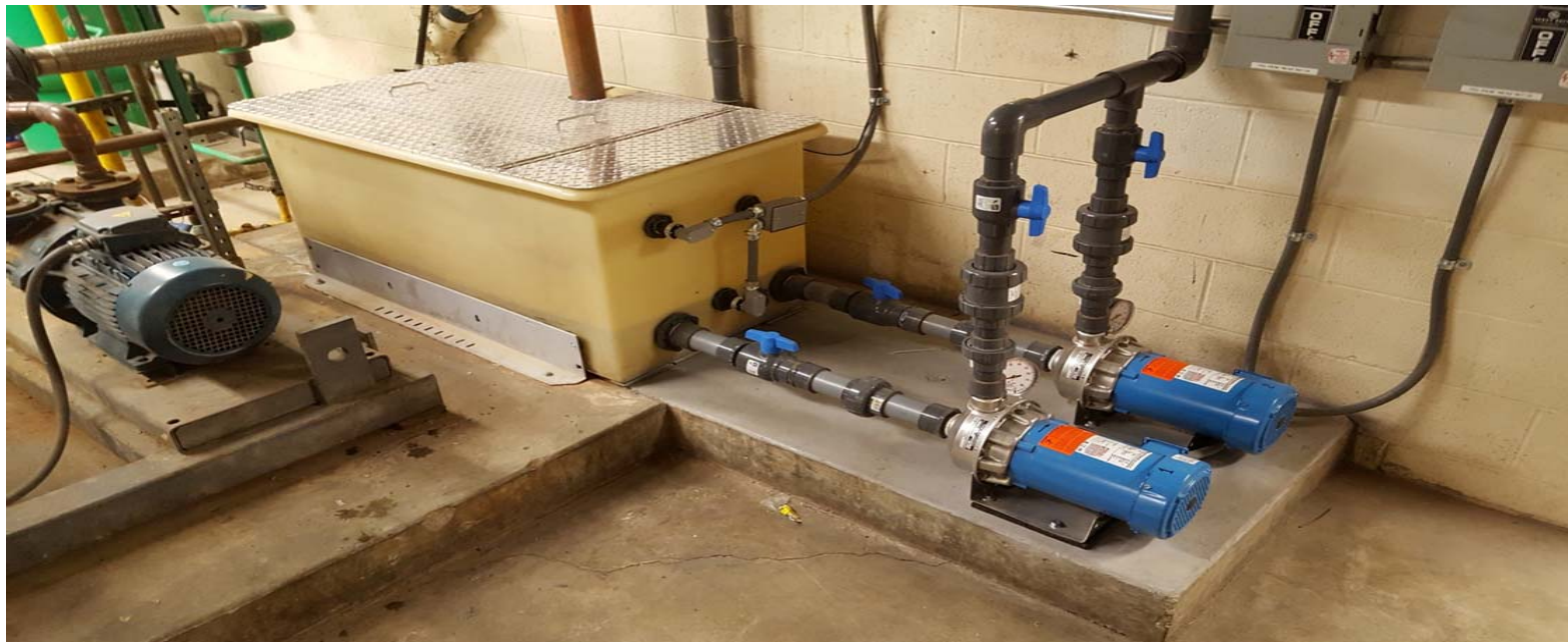
Typical receiver tank
