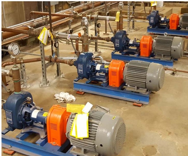
Sump tank pumps
