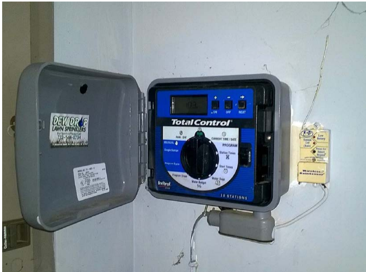
Figure 16: Existing Irrigation Controller Replaced for the Study.
