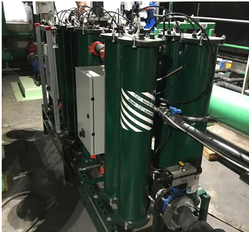
Figure 5. One of two UET reactor skid installations. Photo by Sammy Houssainy
